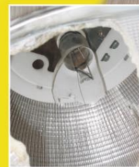
Dangerous result of conventional lamp explosion
